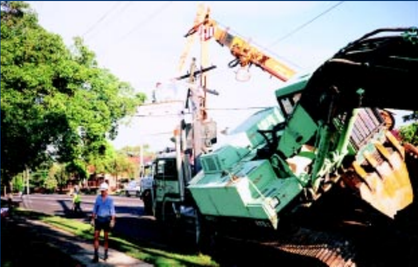
The tracked excavator hit a power pole and slid off the trailer. When carrying high or wide loads always allow for the extra clearance needed to clear obstructions.
